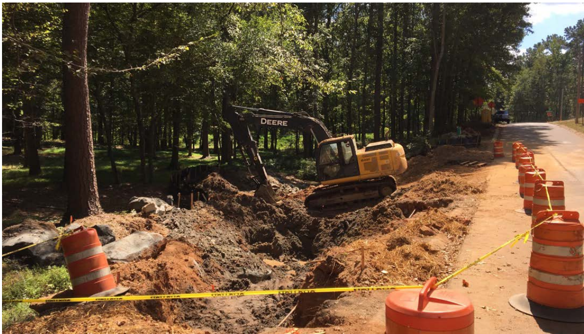
Photo 2: With the large rock removed, waterline relocation activities will resume next week.
