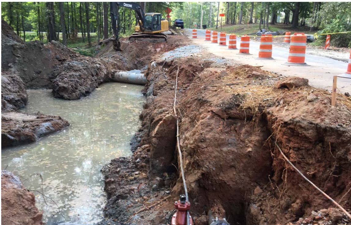
Photo 2: Water began filling the waterline trench on 10/05/2018 and remained in the trench today. Although water was present, work crews were able to install the tapping sleeve.
