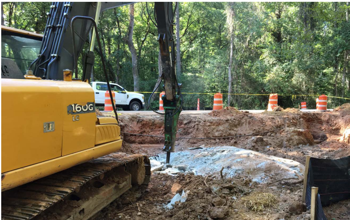
Photo 2: Larger rock breaking equipment arrived on site, and crews began breaking up the rock.
