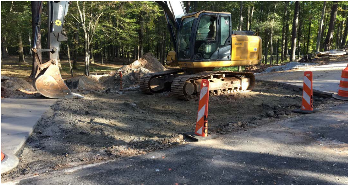
Photo 2: The two regular road lanes have been officially closed. The temporary detour road has been lined with barrels and detour signs uncovered. The asphalt has been cut and removed from the roadway.
