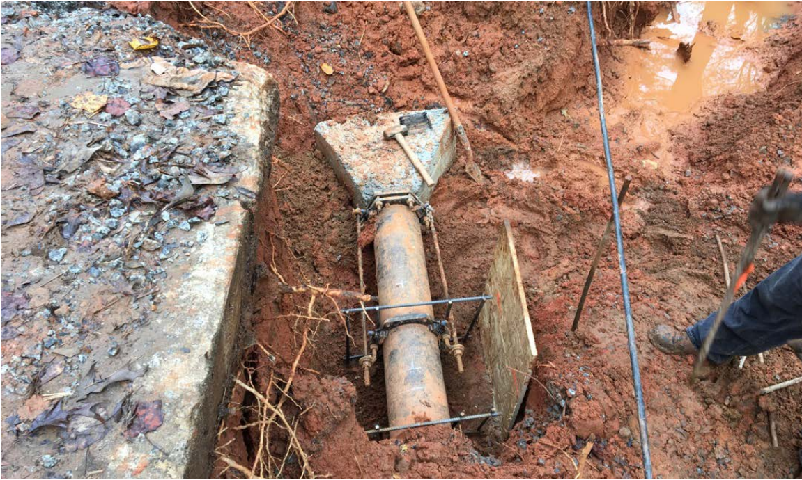
Photo 1: The thrust blocks were placed at the end caps on 11/05/2018. Contractor is constructing forms and placing rebar for the dead man blocking.
