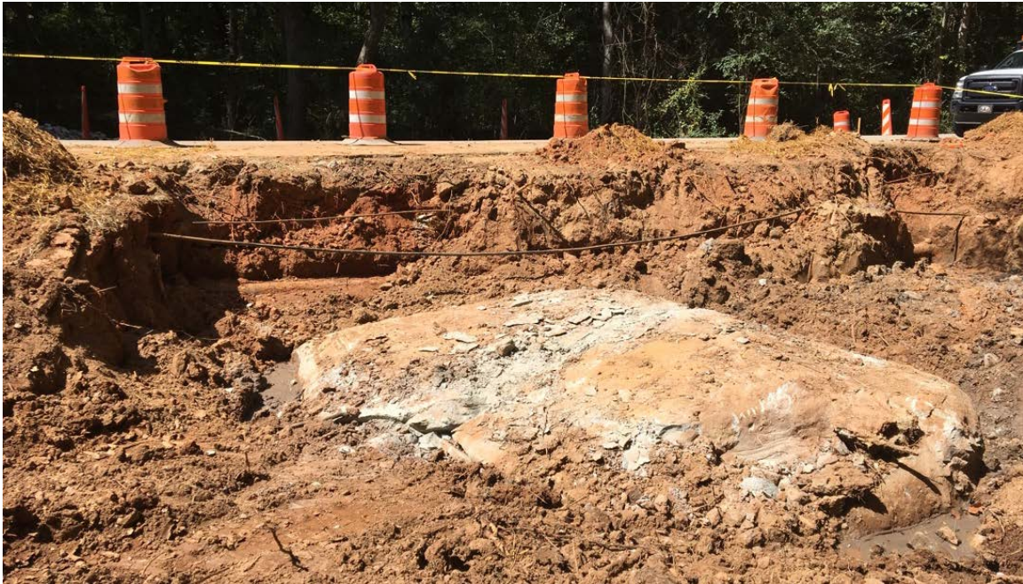
Photo 1: The contractor was not successful using the equipment to demo the rock. Larger rock breaking equipment will be delivered tomorrow.
