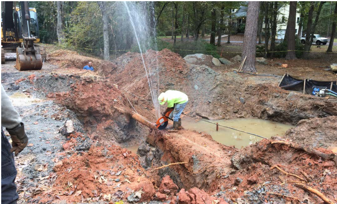
Photo 2: Work resumes on the waterline. The site was prepared with equipment to cut the existing (old) waterline, and materials are on site for capping, rodding, restraining cap to pipe, and concrete block construction. The waterline is cut to relieve pressure and to allowing water drainage.
