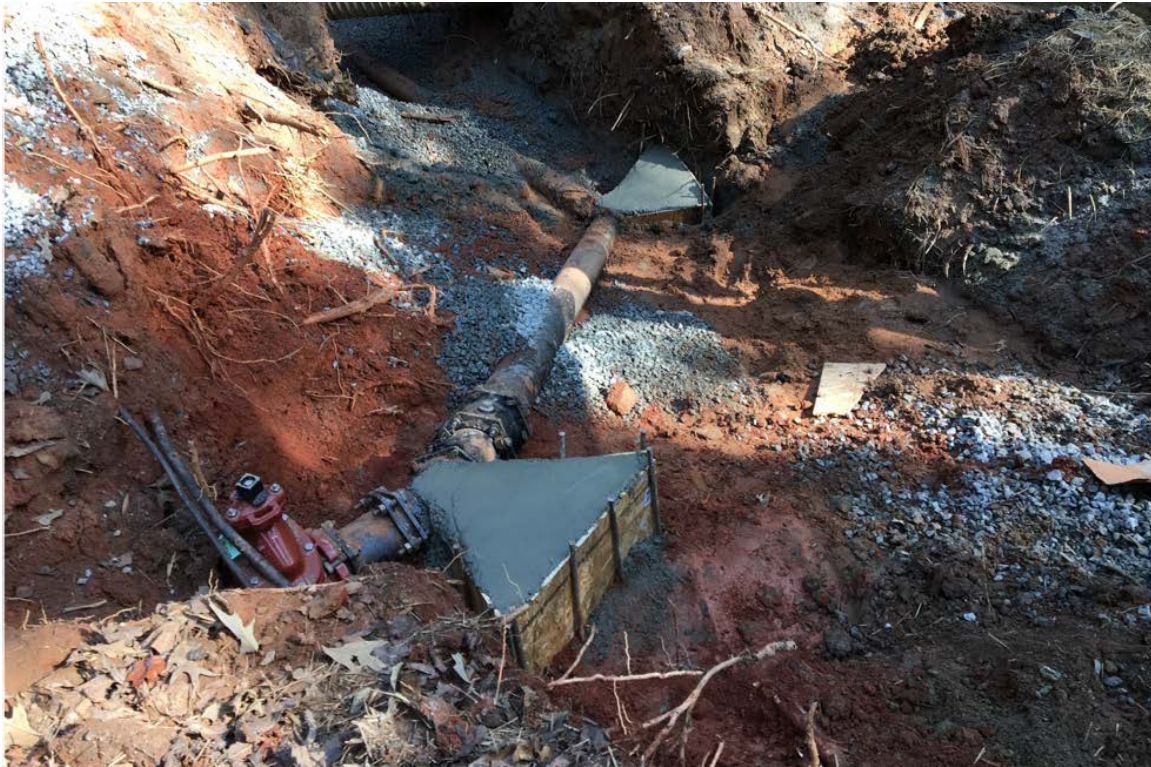
Photo 1: The 8" waterline was flushed and the 8"x2" tapping tee is being installed.
