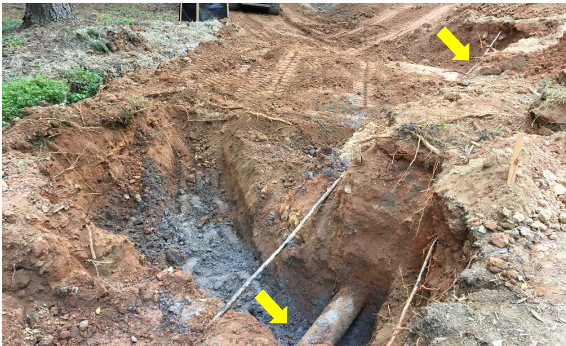
Photo 2: Excavation is complete at both water valve locations (noted above). Excavation for the pipe continues. Installation of pipe and wet taps will begin next week.
