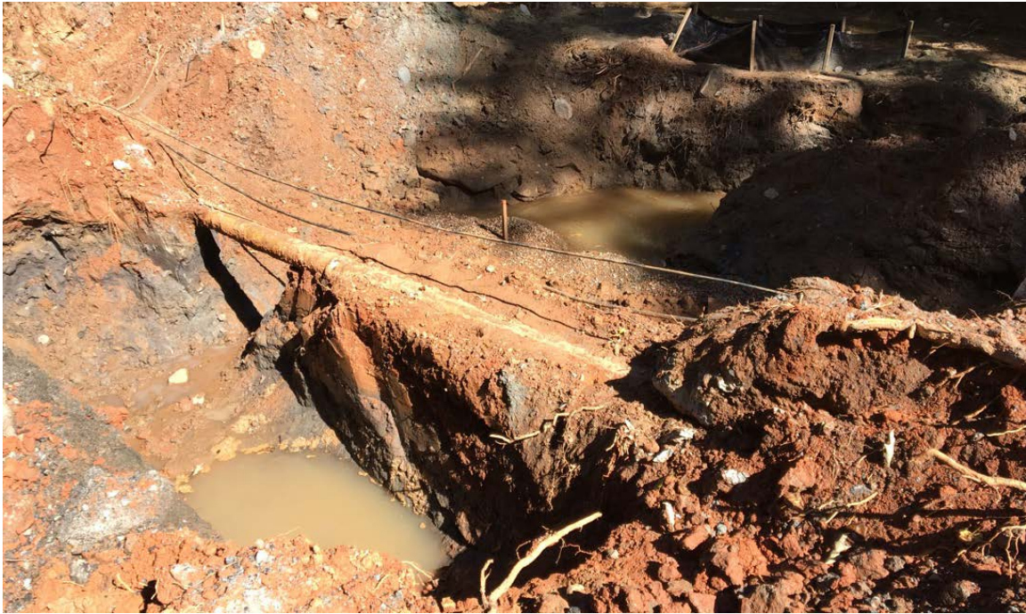
Photo 1: The existing (old) waterline continues to be excavated and exposed. The waterline will be cut and capped, and water service is transferred to the new waterline (tentatively on 11/01/2018). A utility line (thin cable above waterline) remains in the way of the contractor. The utility has been notified, but has not arrived to relocate their utility line.
