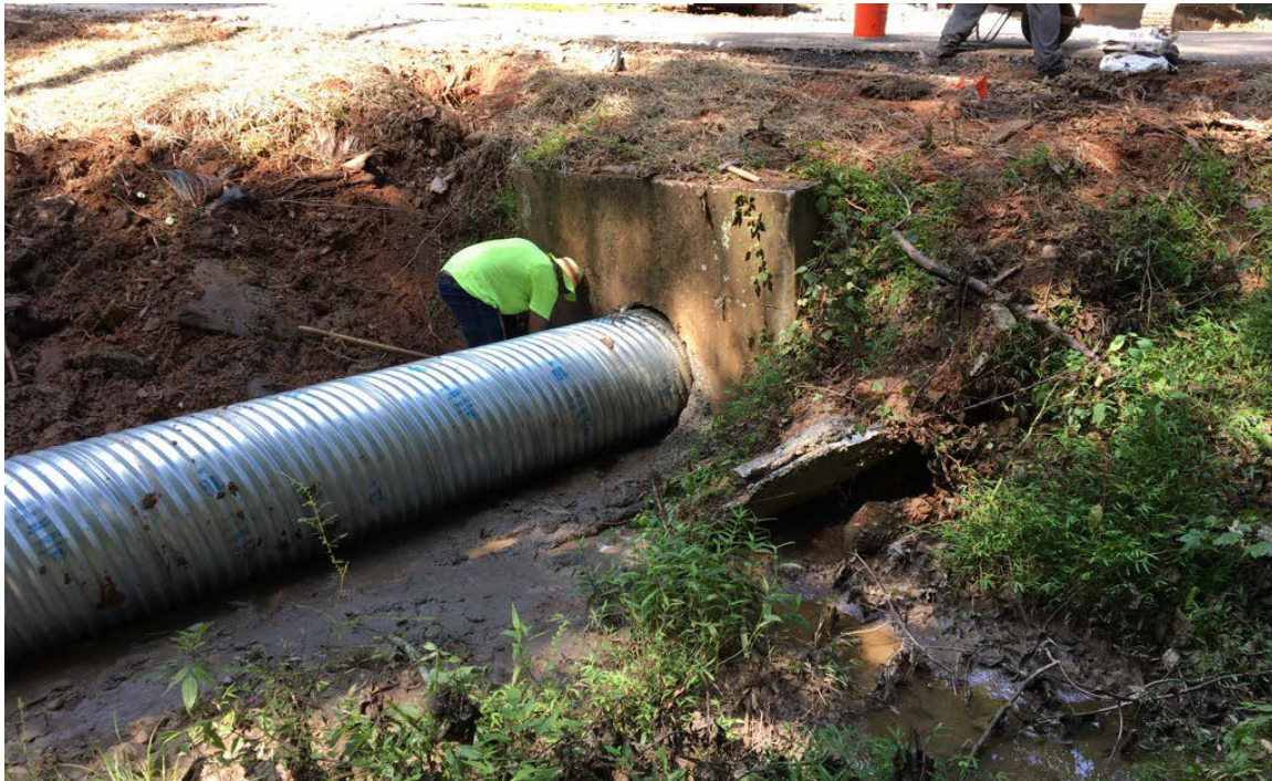
Photo 2: The diversion pipe is installed and the joint is currently being grouted at the existing culvert outlet.
