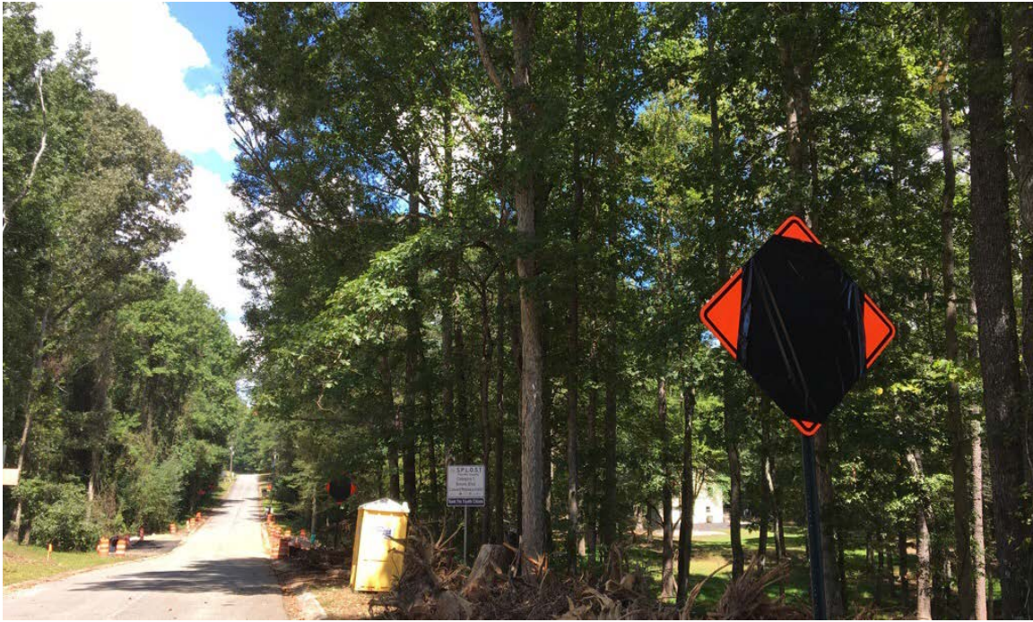
Photo 1: Temporary detour road signs have been installed. They will remain covered until road demolition begins. Waterline relocation is scheduled to begin soon.
