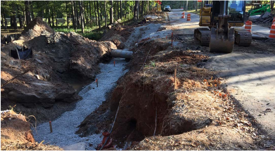
Photo 1: The new waterline passed the pressure test. Gravel is placed in the trench to cover the new waterline. Water service will be shut off in the coming days, to allow transfer of water service from old waterline to new waterline.
