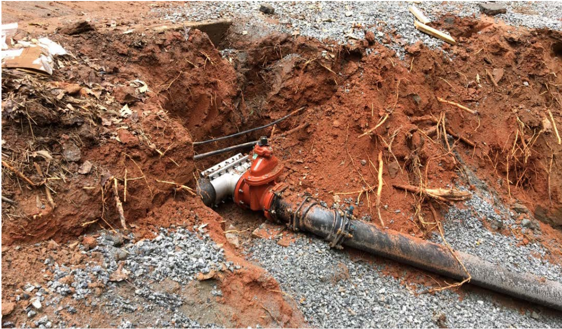
Photo 1: Final piece of pipe has been installed. **Work delayed for two days due to anticipated severe weather related to Hurricane Michael.
