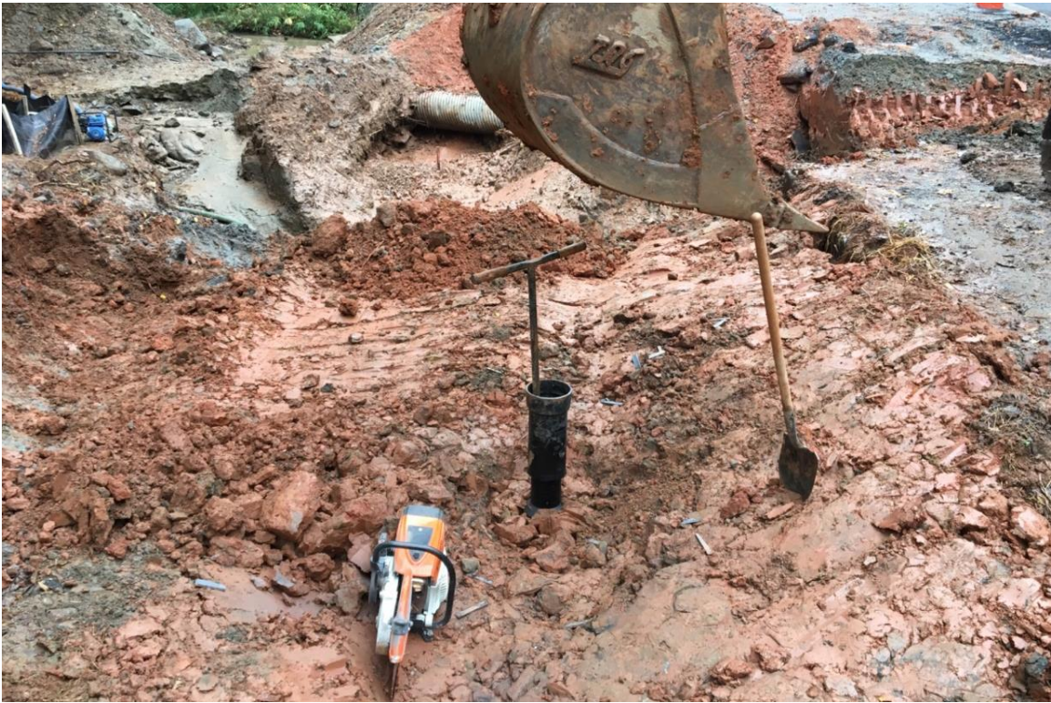
Details: Deadman blocking completed, valve sleeve placed, and backfilled at both waterline valve locations.
