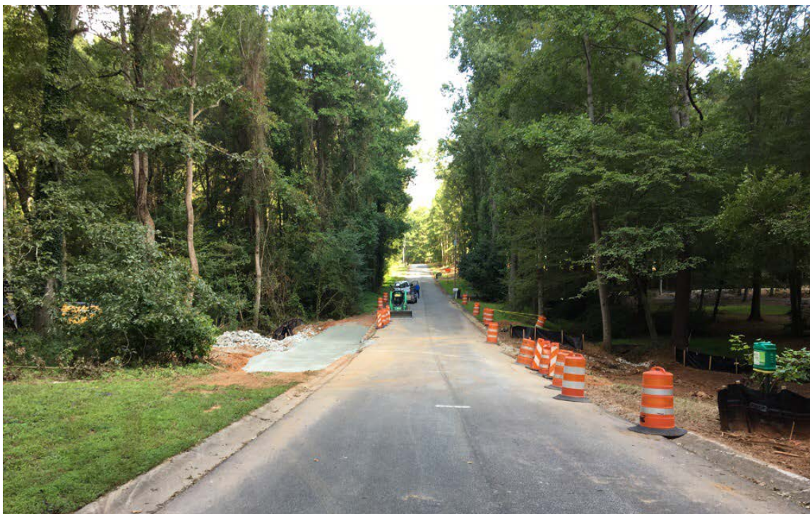
Photo 2: Overall site view. Additional GAB will be delivered for the temporary detour road and asphalt placement will follow.
