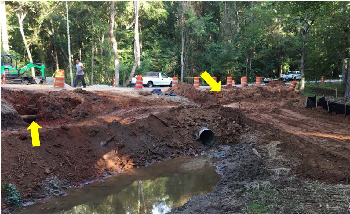
Photo 1: Excavation is complete at both water valve locations (noted above). Excavation for the pipe continues. Installation of pipe and wet taps will begin next week.
