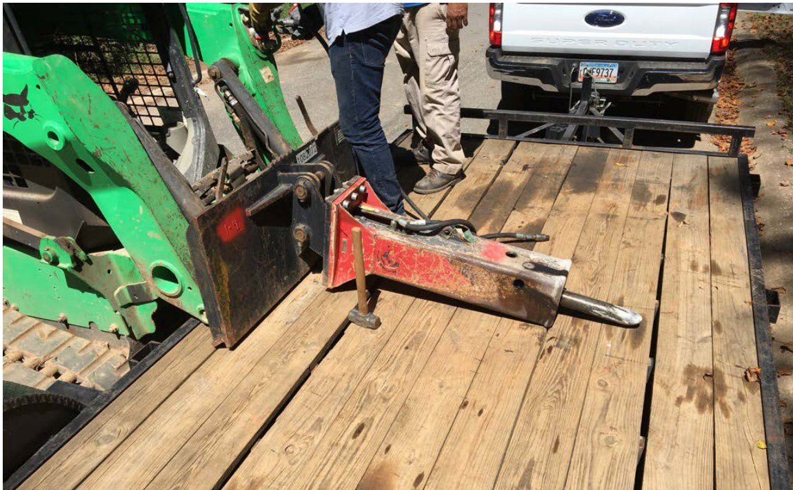
Photo 2: Special equipment arrives at the work site, to assist with breaking up the rock.
