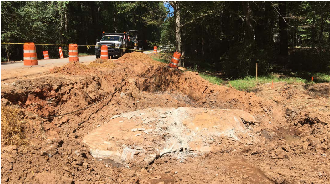
Photo 2: The contractor was not successful using the equipment to demo the rock. Larger rock breaking equipment will be delivered tomorrow.
