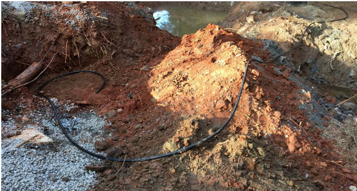
Photo 2: AT&T has placed a new communication line (black utility line visible in photo above) in the construction area, but it was not connected or buried today.
