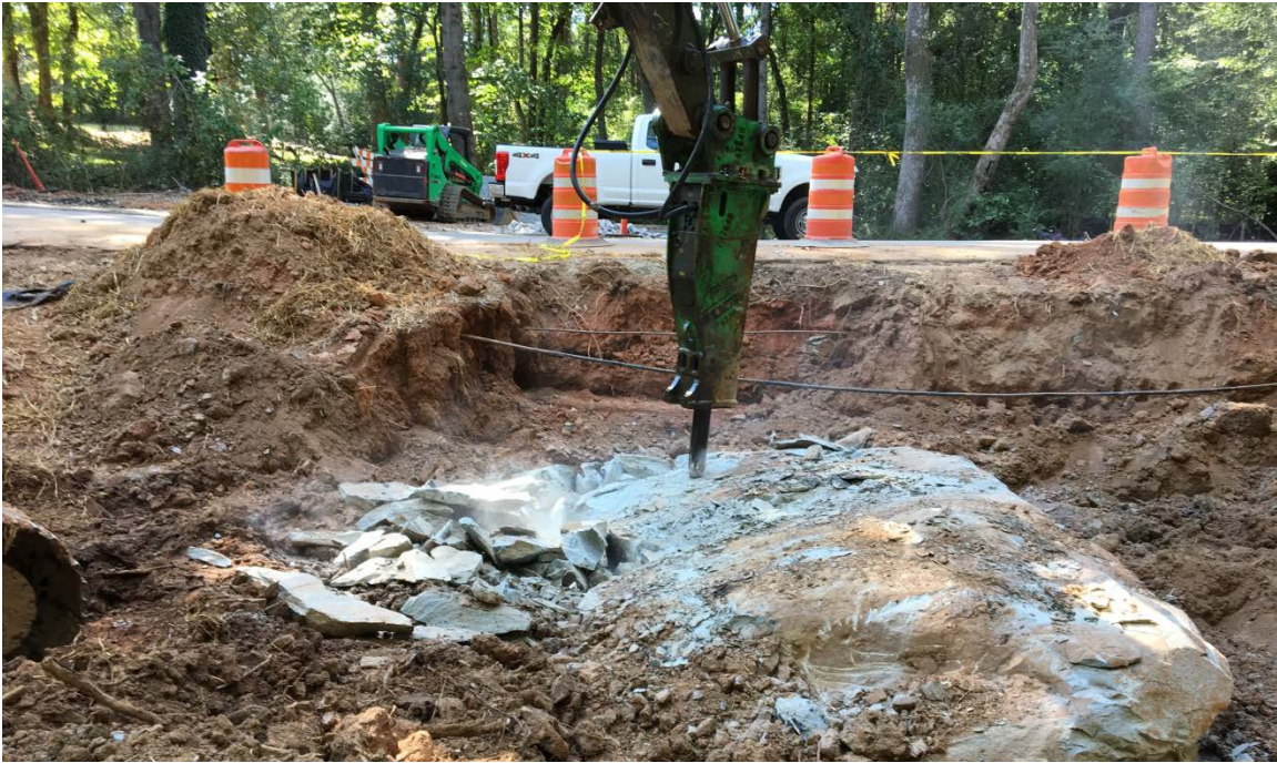
Photo 1: The rock debris will be removed from the site, once the demo is complete.
