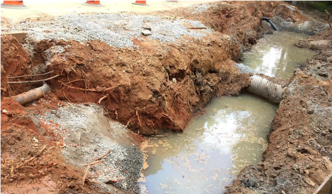
Photo 1: Water began filling the waterline trench on 10/05/2018 and remained in the trench today. Although water was present, work crews were able to install the tapping sleeve.
