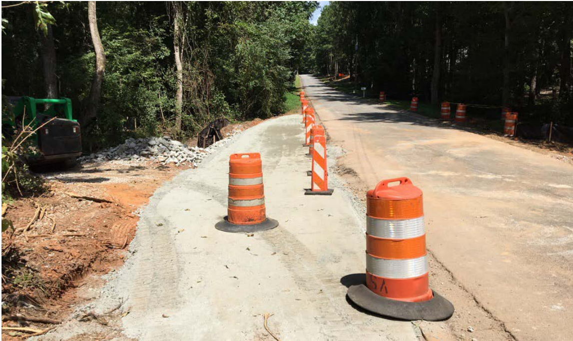
Photo 1: Construction of the temporary detour road continues. Additional GAB has been delivered and installed. Asphalt will be placed soon.
