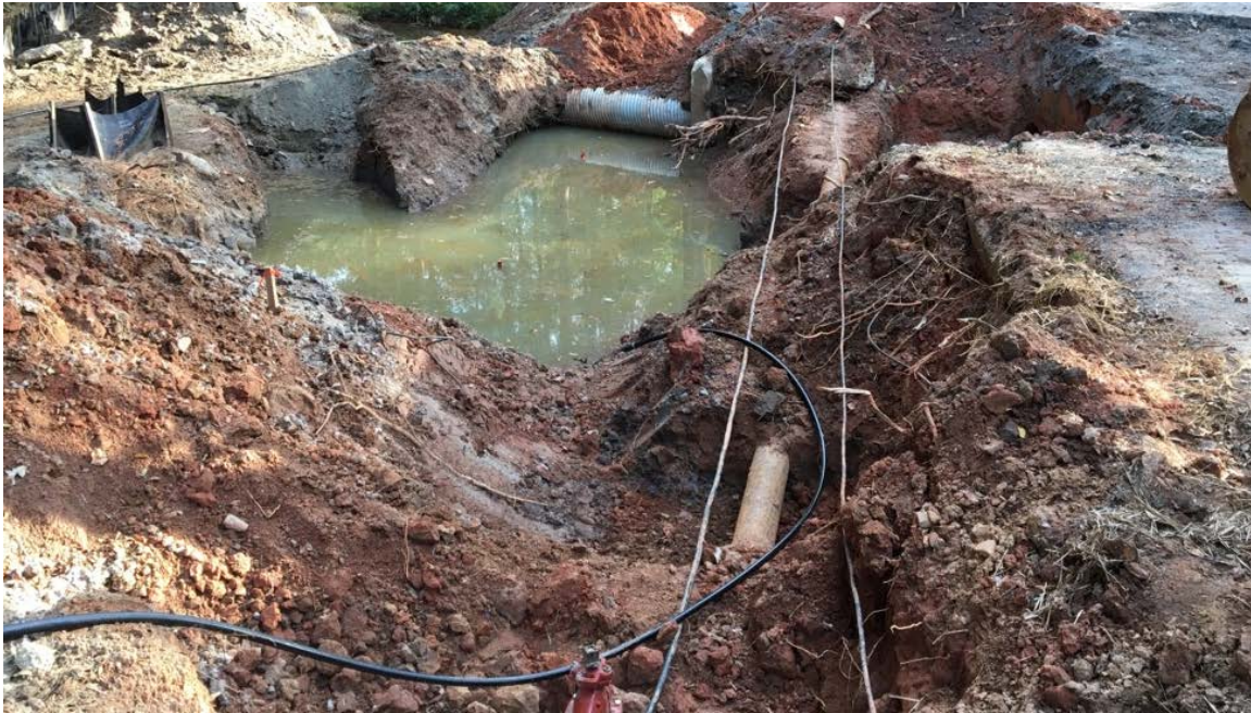
Photo 1: Work was not performed the previous day to allow soil to dry. Site conditions are still wet and halted work today.
