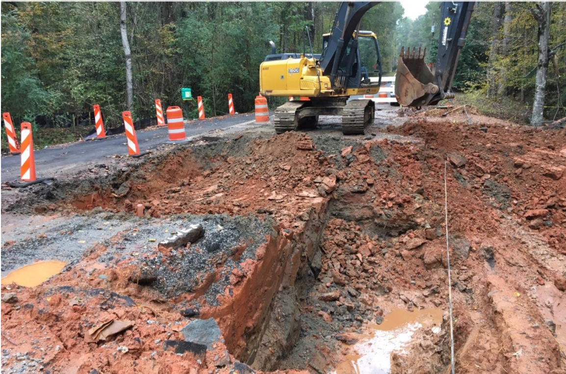
Details: Excavation continues within the existing road area. Soil testing scheduled for the following day.
