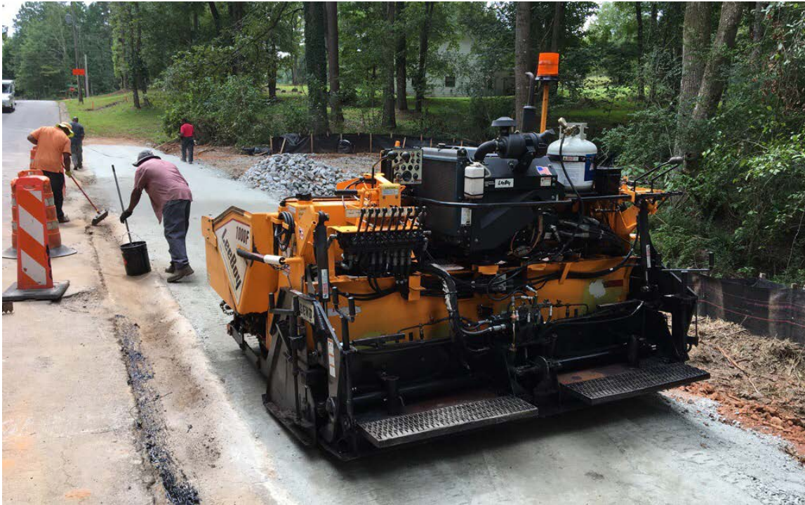
Photo 1: Construction of the temporary detour road continues. Asphalt paving is underway and contractor expects it to be complete by the end of the day.
