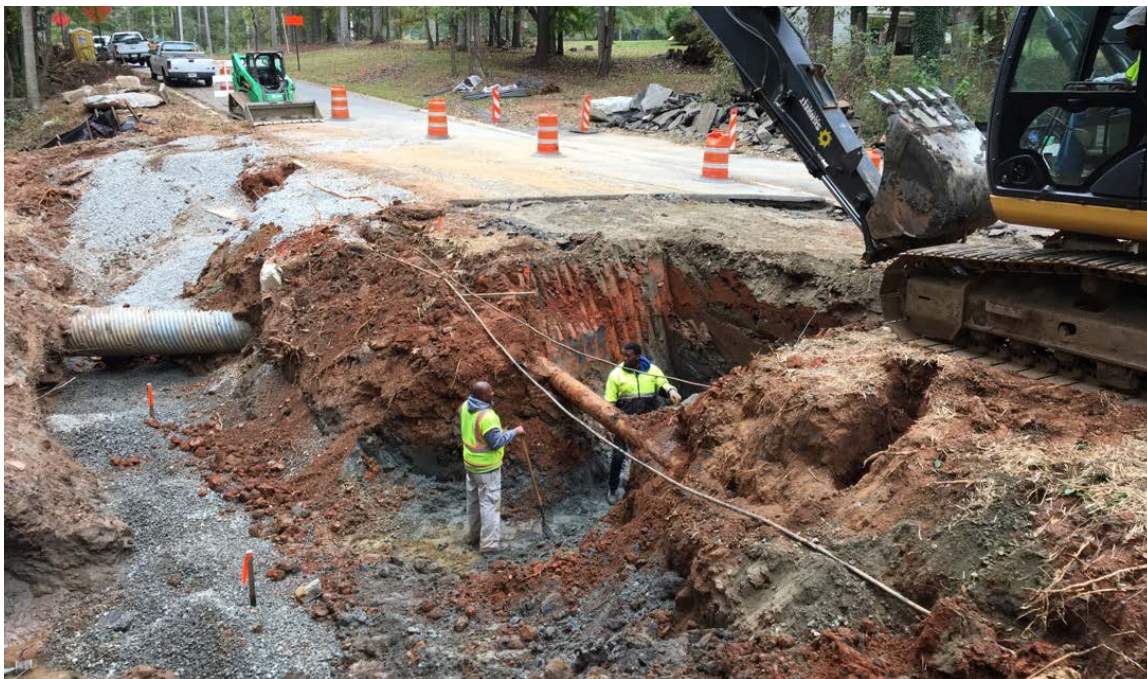
Photo 2: The area below the asphalt cut and removal is being excavated. The existing (old) waterline is exposed. The waterline will be cut and capped, once the water service is transferred to the new waterline.
