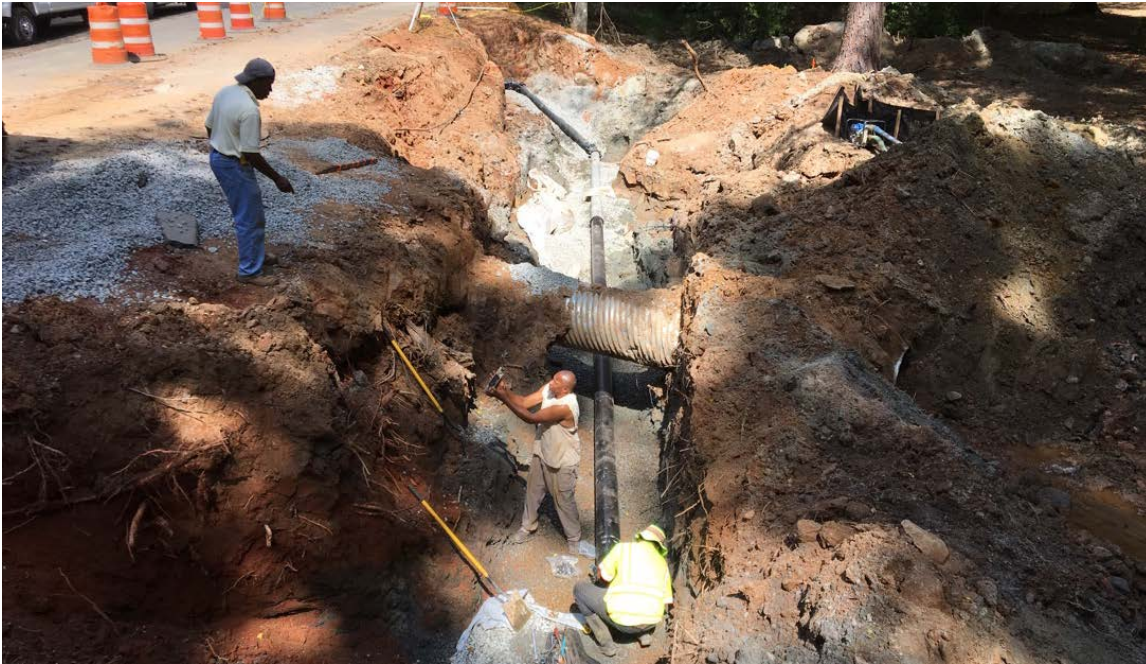
Photo 1: Installation of the 45 degree pipe fitting is in progress and will be followed by tapping sleeve and water tap installation in the coming days.
