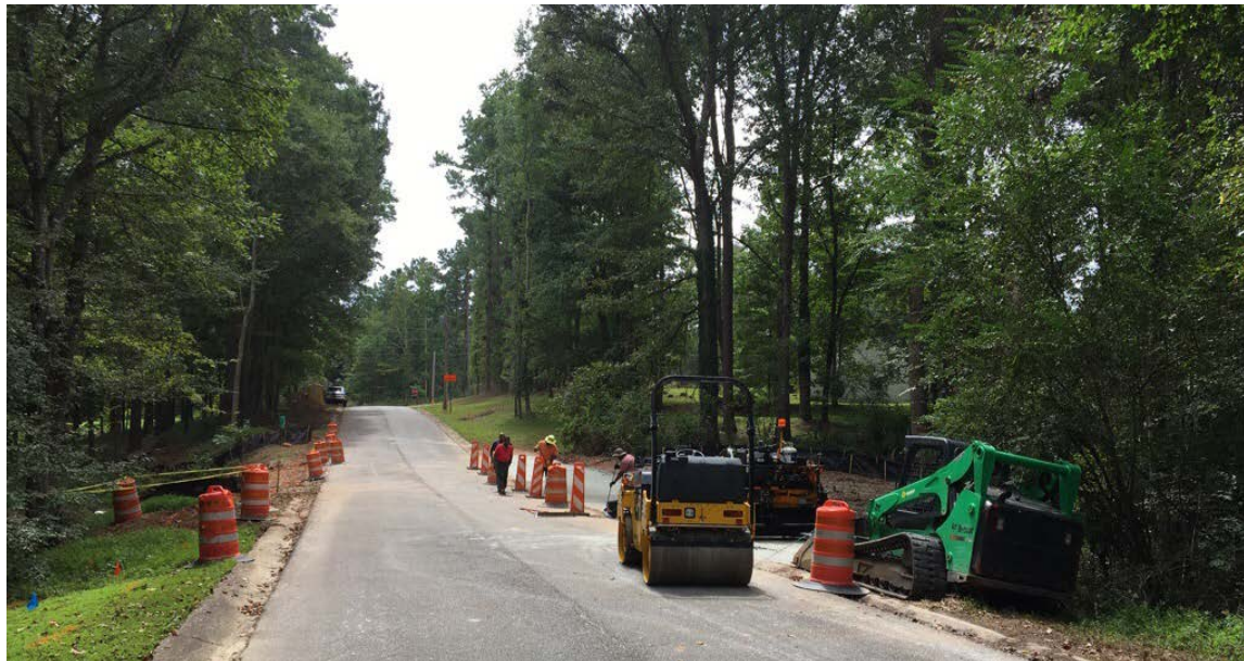
Photo 2: Construction of the temporary detour road continues. Asphalt paving is underway and contractor expects it to be complete by the end of the day.
