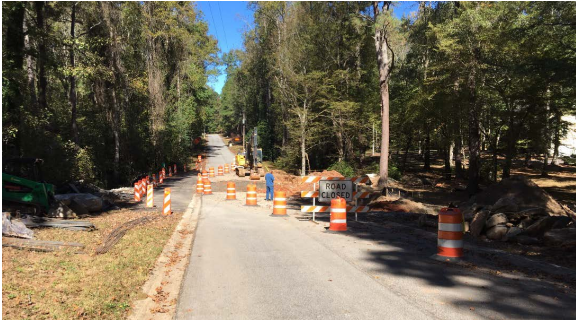
Photo 2: Overall site condition. Temporary detour lane is lined with barrels on the left side of Broom Boulevard. Work will not be performed tomorrow to allow soil to dry.
