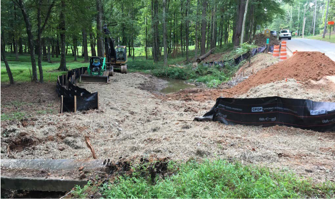
Photo 1: Disturbed areas near the existing culvert outlet have been stabilized with grass seed and hay.
