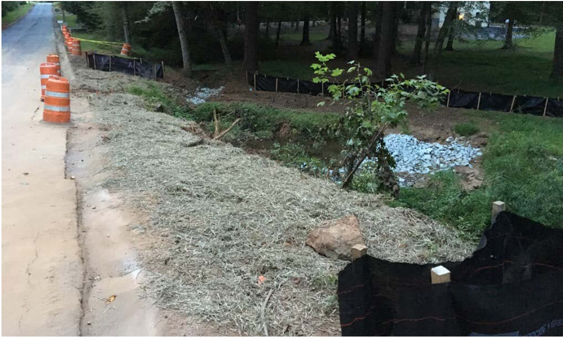
Photo 1: The disturbed areas on the east shoulder of Broom Boulevard are covered with mulch/hay/grass.
