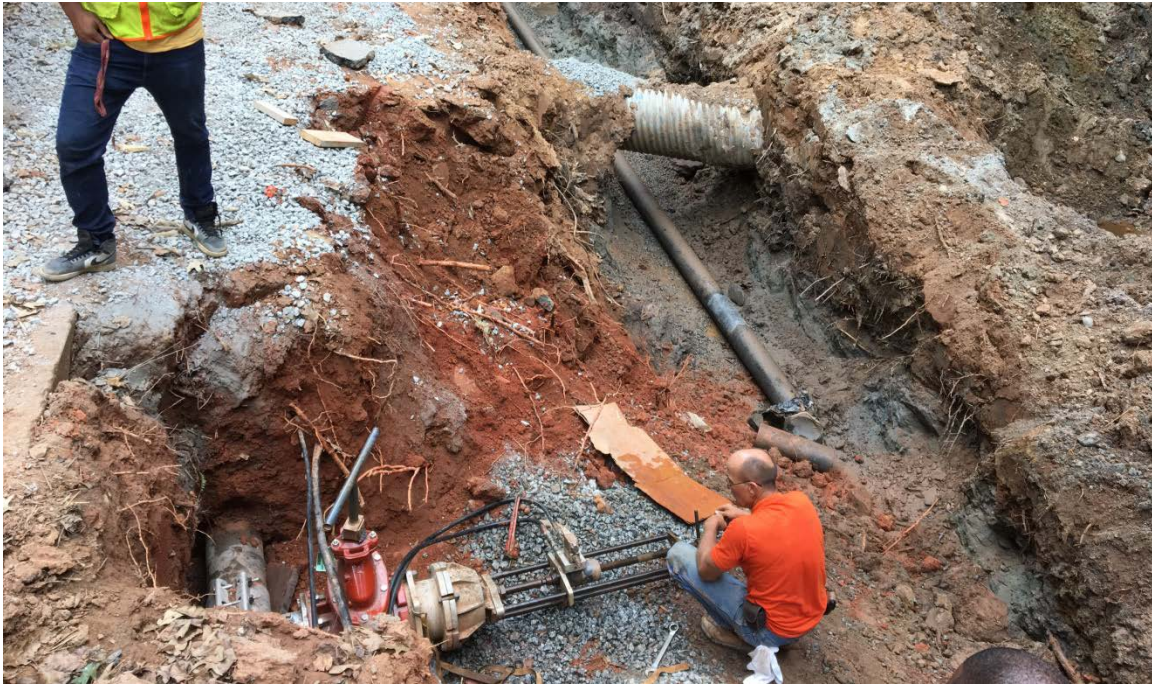
Photo 1: A pressure tests were completed on the tapping sleeve and wet tap. Fayette County was on location for testing. The waterline is now in service.
