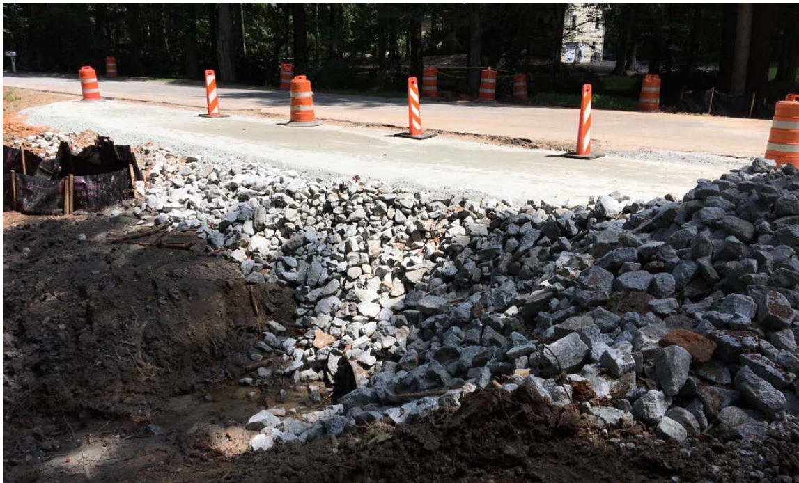
Photo 2: Construction of the temporary detour road continues. Additional GAB has been delivered and installed. Asphalt will be placed soon.
