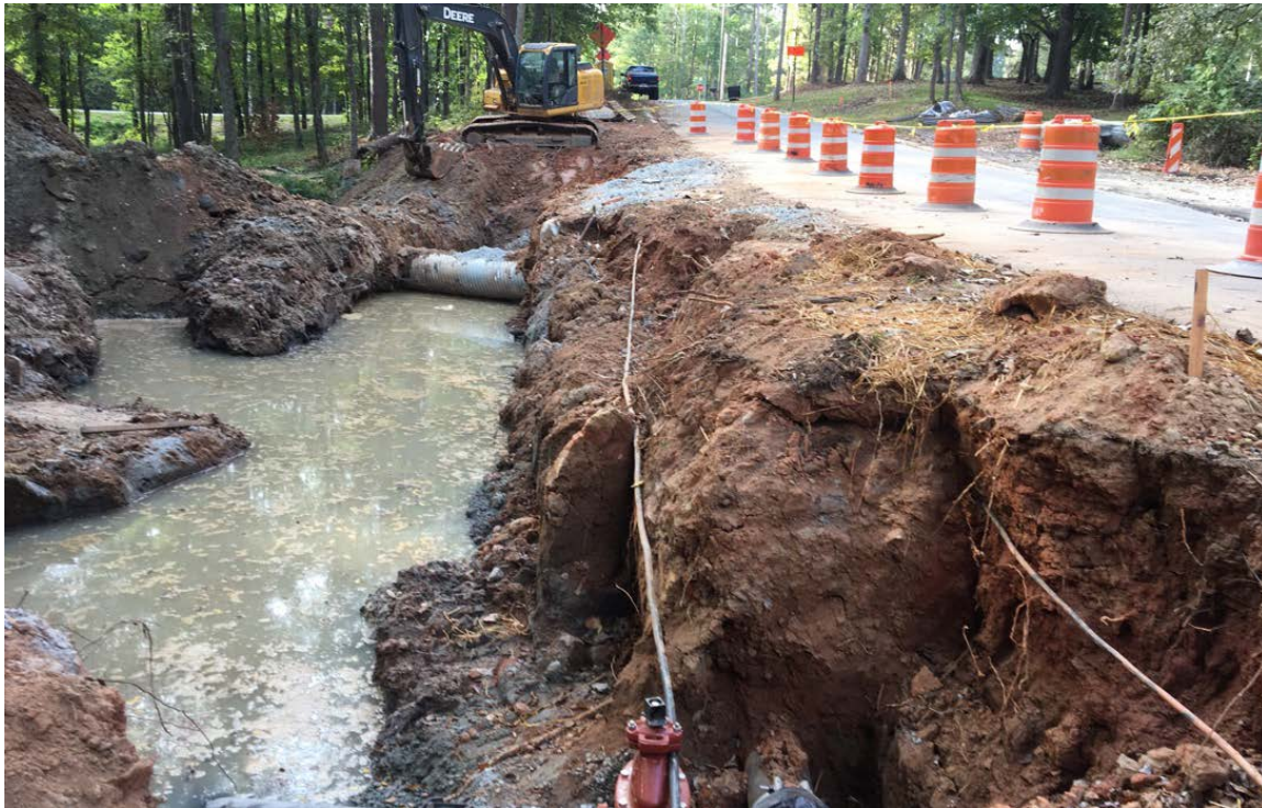
Photo 2: A pressure tests were completed on the tapping sleeve and wet tap. Fayette County was on location for testing. The waterline is now in service.
