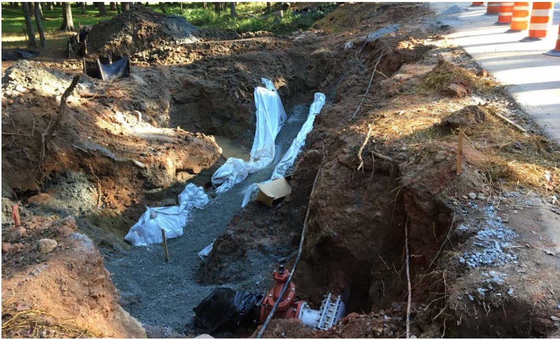
Photo 1: Excavation for new waterline pipe continues. The site for the new pipe has been prepped with a plastic liner and gravel.
