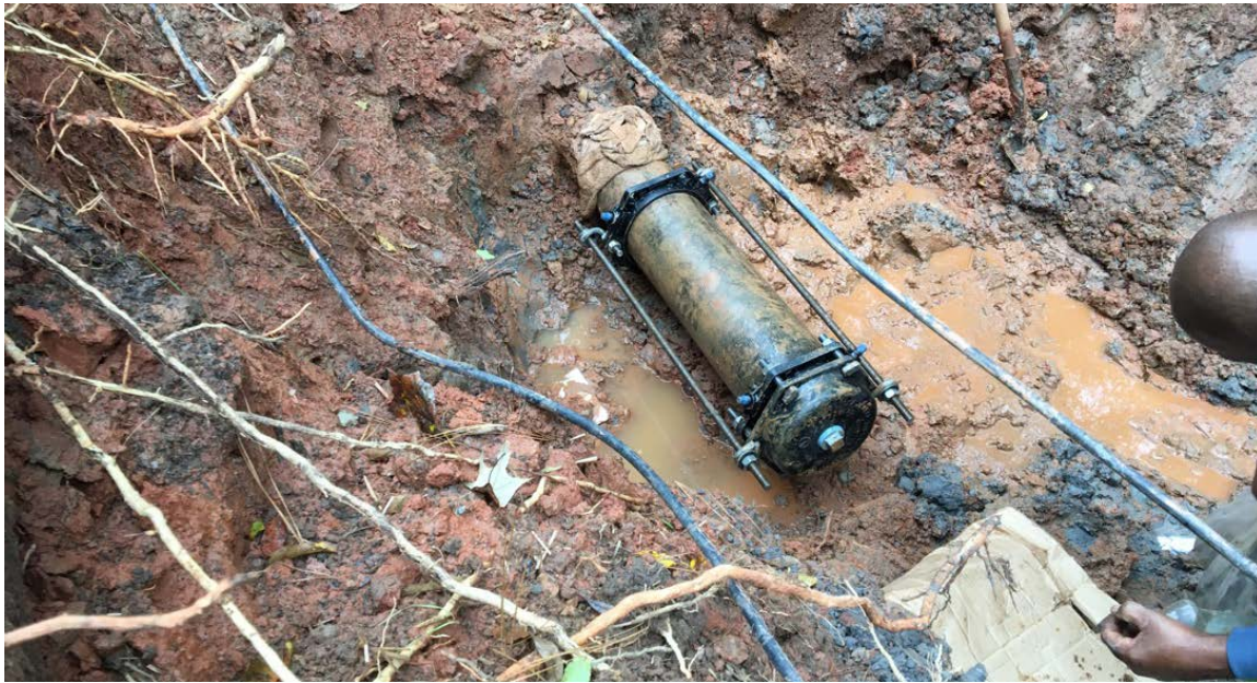
Photo 2: The ends of the existing (old) waterline are capped, after a portion of the pipe was cut and removed. Leak test are in progress. Service is expected to be restored by the end of the day.
