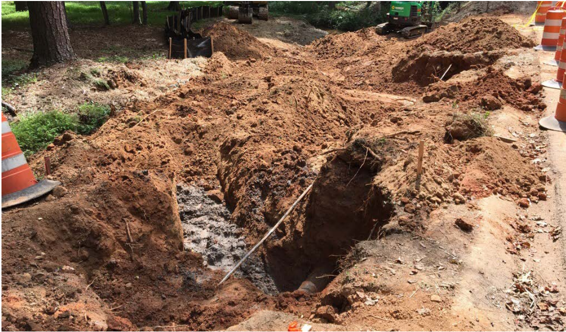
Photo 1: Excavation continues for upcoming waterline relocation. Crews are working around the rock, until it can be removed.
