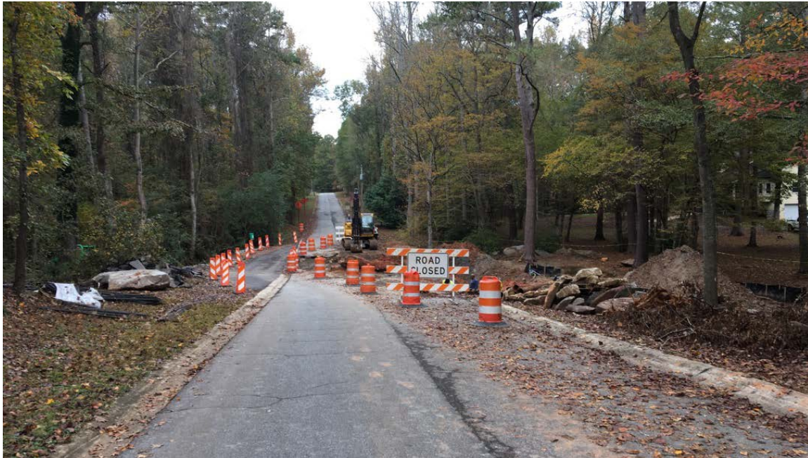
Photo 2: Overall site conditions. Work has been intermittent over the last several days and continues through the coming days due to rain. Today, the work noted above was accomplished; however, no other construction tasks were undergone due to expected rain.
