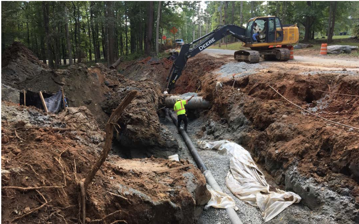
Photo 2: Pipe installation continues and is nearing the tie in location. Approximately 56 feet has been installed.
