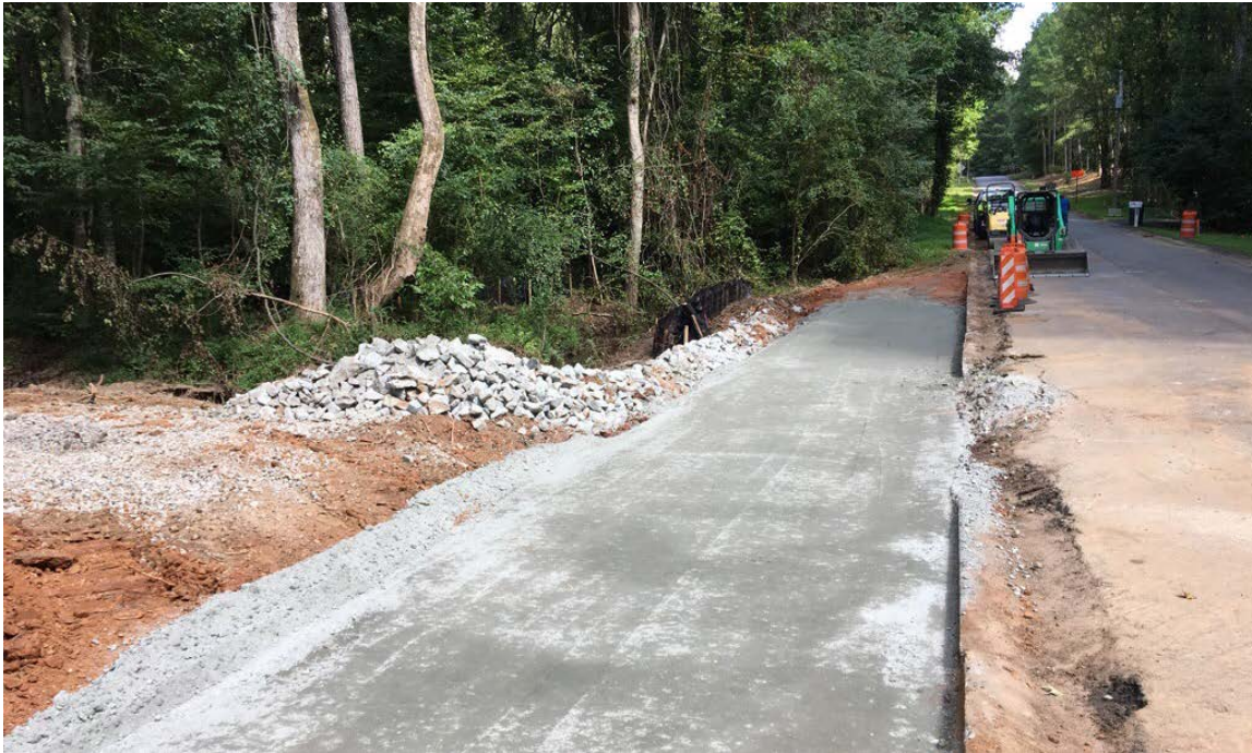
Photo 1: Construction of the temporary detour road continues. Subgrade has been compacted, first layer of GAB placed, and riprap placed between detour road and creek.
