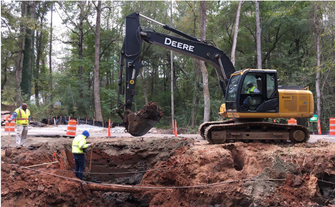
Photo 1: The area below the asphalt cut and removal is being excavated. The existing (old) waterline is exposed. The waterline will be cut and capped, once the water service is transferred to the new waterline.
